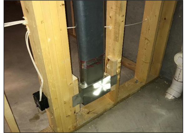
10. Ducted and sealed return air.
